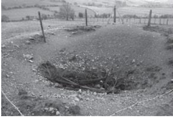
Plate 3.0 A coned mineshaft.
